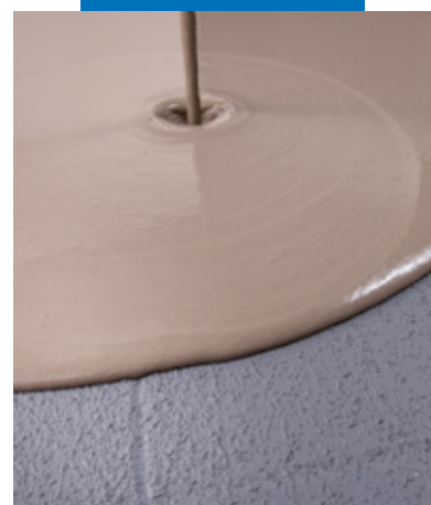
Application of Ultraplan self-levelling smoothing compound on dry Eco Prim Grip on old floor
